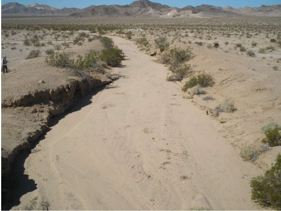
Exhibit I21. 60-foot wide wash, on west side of trestle, facing west towards Chubbuck.
